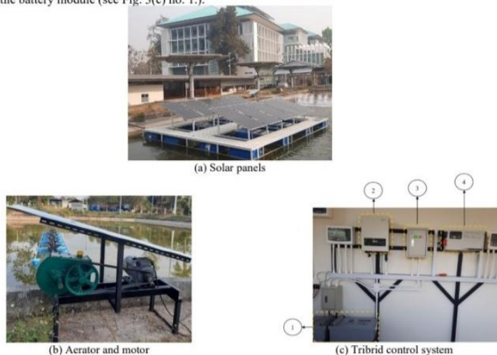
FIGURE 3. The solar aerator with the tribrid power system.
