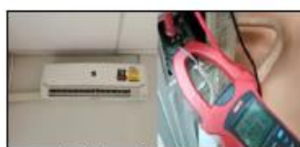
(a) Air conditioning system.
